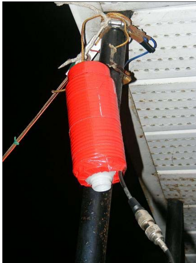
The VE2ITZ Balun with Sloper Antenna!
